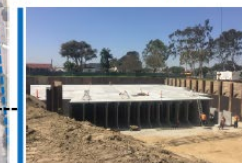
Pre-Cast Subsurface Infiltration Facility
