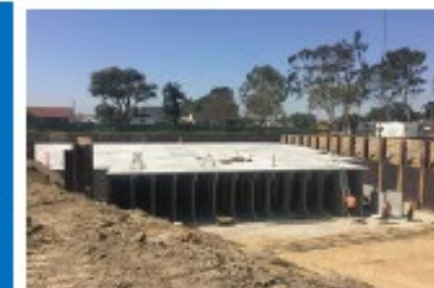
Pre-Cast Subsurface Infiltration Facility
